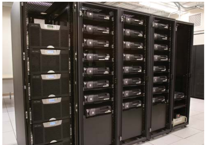
The BladeUPS remains cool even in a data center full of servers.
